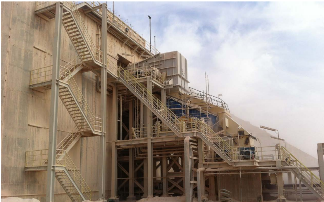
Figure 17-3: Typical above ground crushing facility
